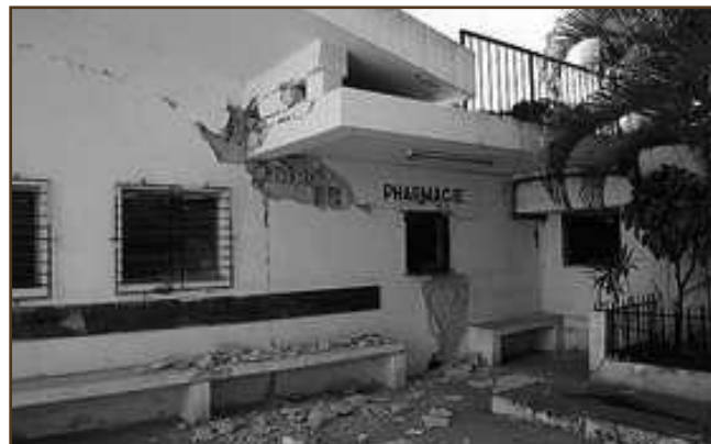
One section of Hospital Ste. Croix damaged in the Haiti earthquake.
