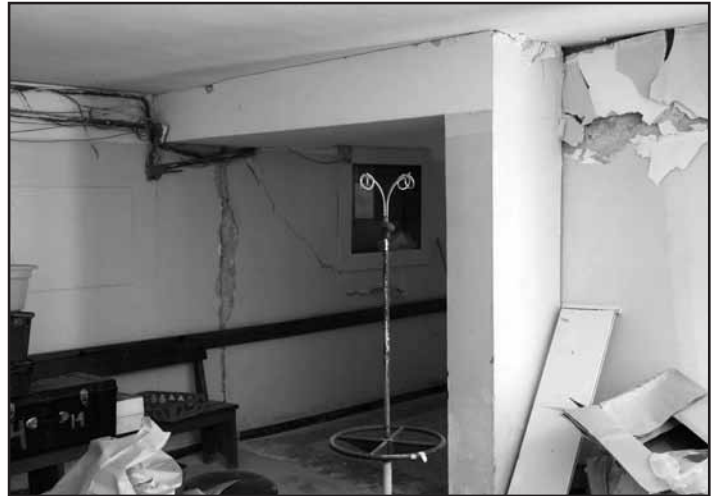
Interior of one of the hospital rooms after the earthquake.
